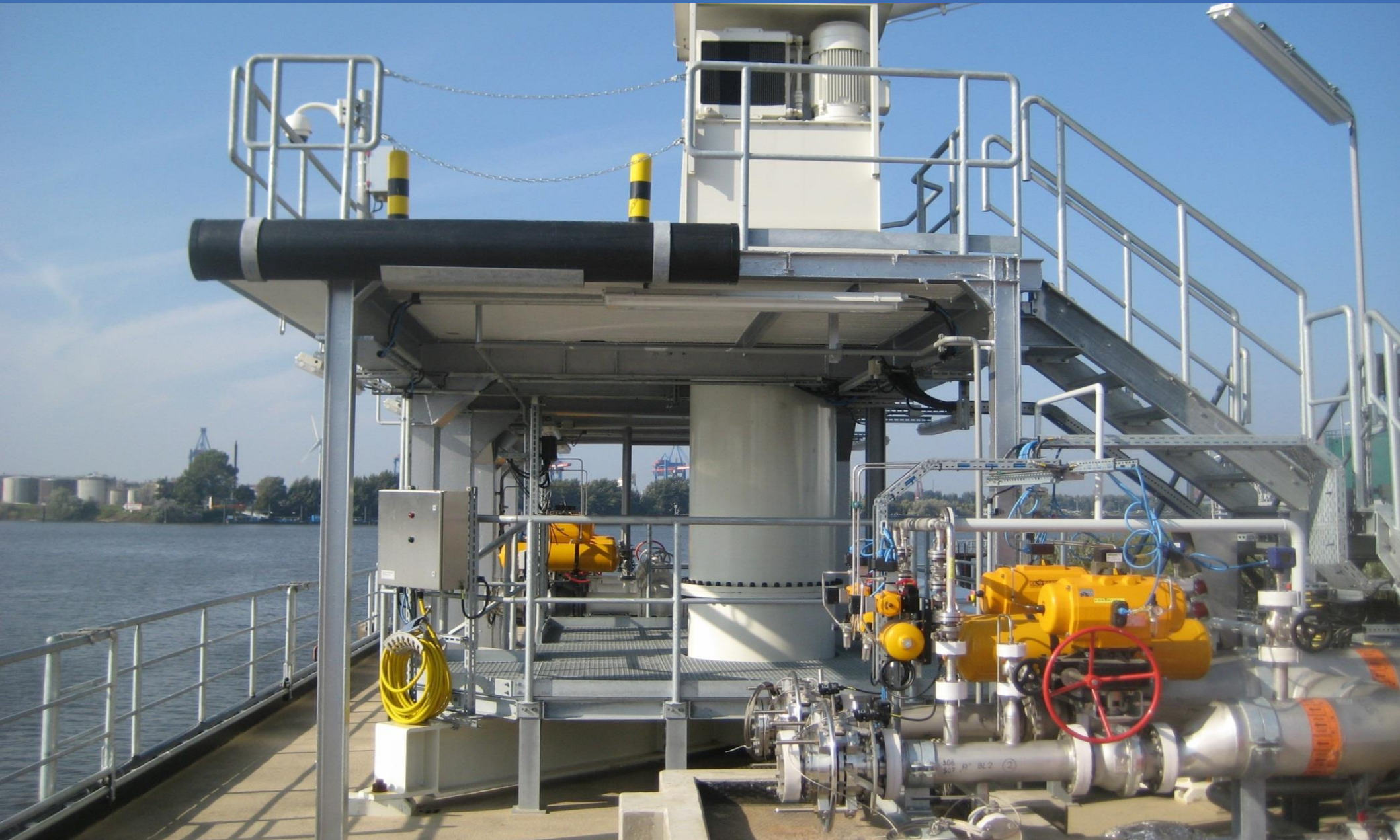
Loading Dock with Marine Grounding System SEK-2
